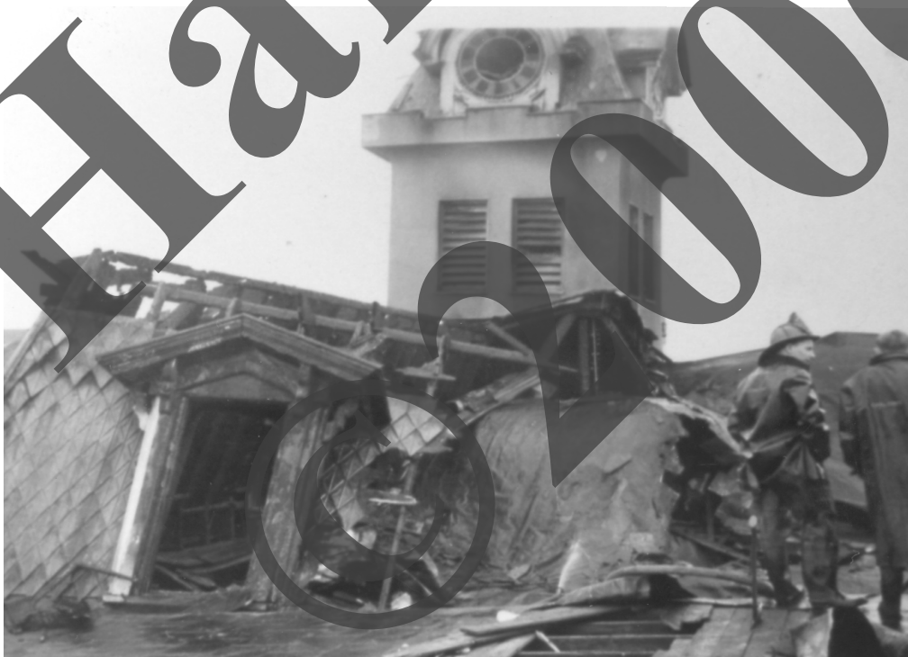
Fire damage to the upper story and the tower.
