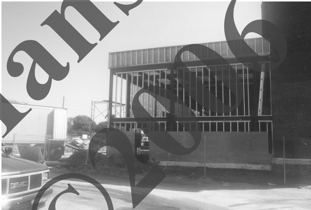
A large extension was added to the rear of the theater to provide space for dressing rooms, storage space for stage props and equipment and a loading ramp.
