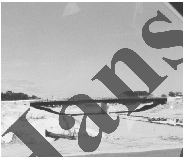
The North Ocean Avenue bridge under construction, June 1989. The reconstruction of Sunrise Highway, to turn it into a limited access highway, began in 1988 on the Nichols Road to Phyllis Drive section. Again this section was started before the Oakdale to Sayville section
