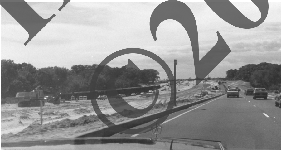
This picture of Sunrise Highway under construction was taken in 1989 from the North Ocean Avenue crossing looking west. The Waverly Avenue bridge, under construction, can be seen in the distance.
